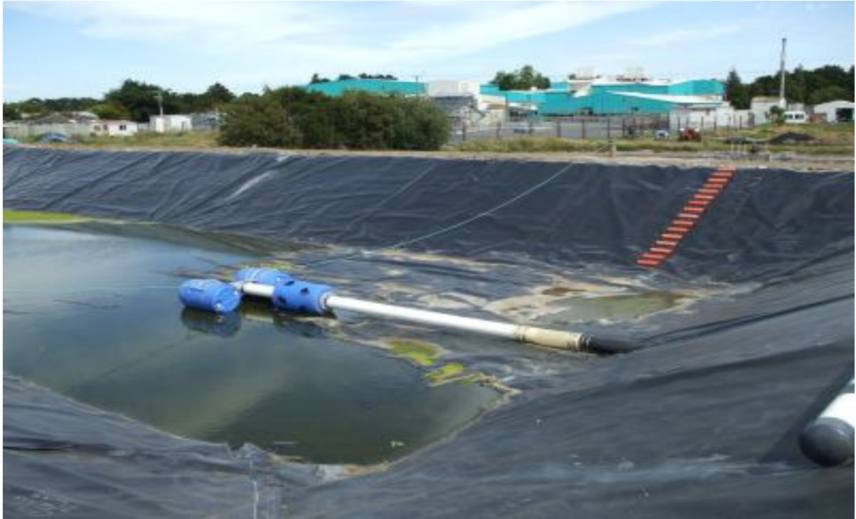
Waste Water Pond.
